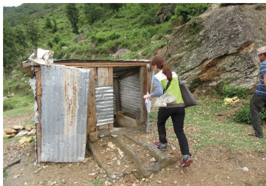
Fig. 4. A make-shift toilet in Nabadurga Bhawani Basic School, Bajura district.
